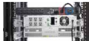
HotSwap MBPs rackmounted horizontally in rack
